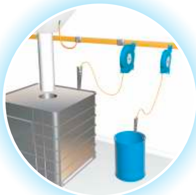
Grounding of metal IBCs and drums with clamps and retractable reels (more detail overleaf)
